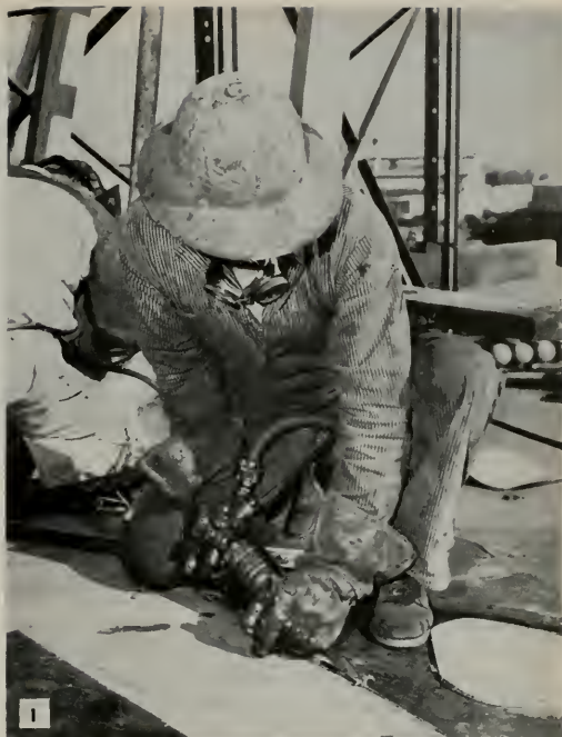
Fig. 1—Grooving of main deck plates for welding goes faster and more economically at the National Iron Works shipyard with the aid of compressed air-operated chipping hammer. The work is being done on the "Ruthie B," new 110-foot tuna boat.
